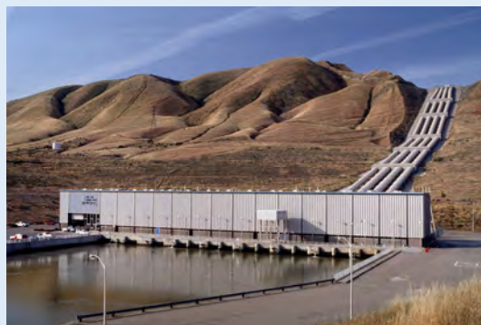
State Water Project (SWP) Chrisman Pumping Plant. Credit: DWR
