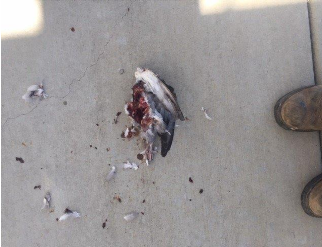
Photo 15. Dead pigeon carcass as observed by LEC personnel under CTG Generator breaker. April 15, 2018.
