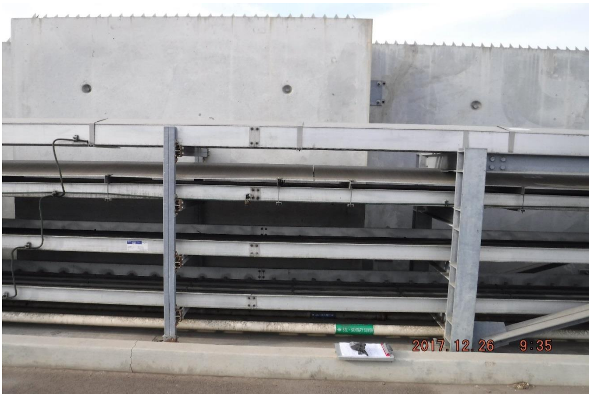
Figure 1. Cable rack and location of the two nests.
