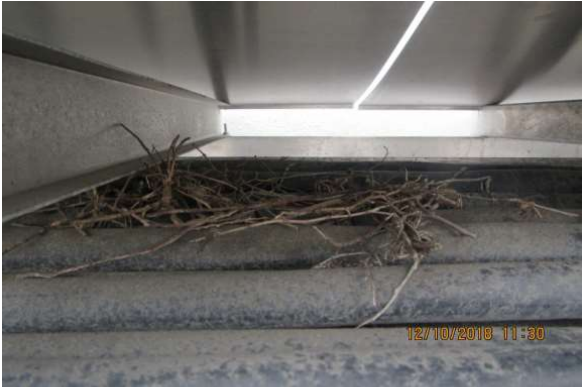
Figure 3. Poorly constructed nest, adjacent to that shown in Figure 2.
