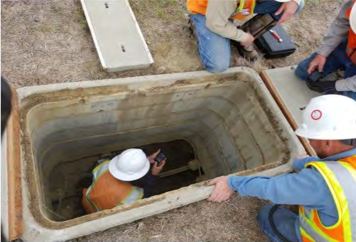
Photo 9, of waterline vault work to facilitate addition of self-cleaning screens at canal pumps, 4/10/18.
