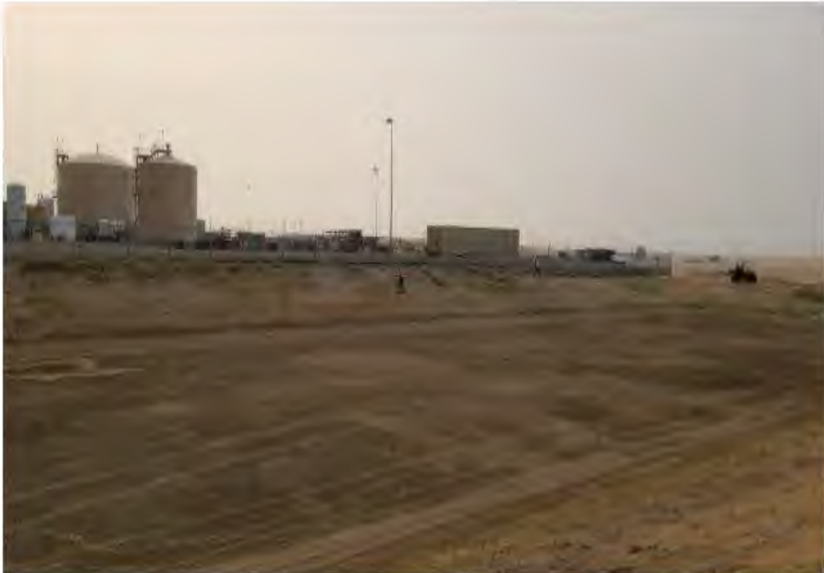
Photo 59, of vegetation clearing on edges of CGS detention basin for wildfire protection, 8/8/18.
