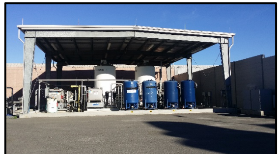
RO Skid Structure (1/24/19)
