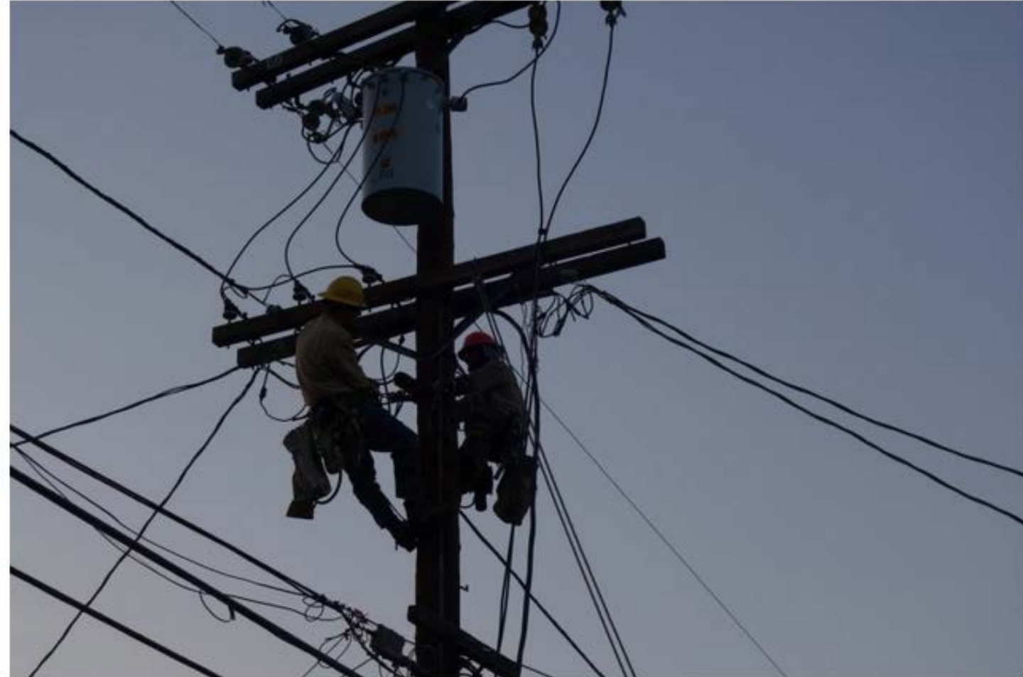
Line crews with the Los Angeles Department of Water and Power, seen here atop a pole replacing a transformer on Sunday, July 8, 2018, work to restore power to thousands during the weekend's heat wave in the region. (Photo courtesy LADWP via Twitter)
