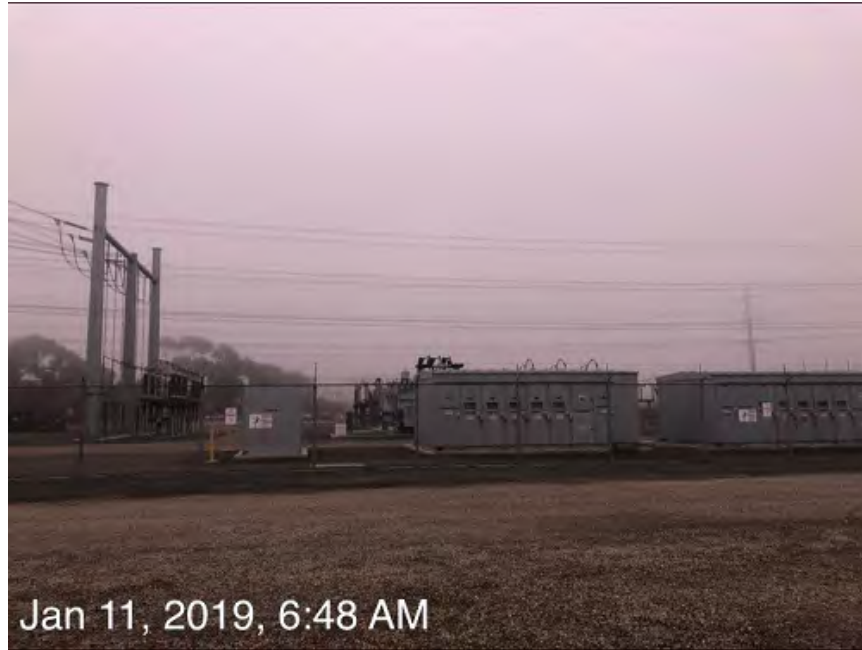
Photo 7. The Canon Substation was surveyed for biological constraints and none were identified. Photo taken 1/11/19, facing south.
