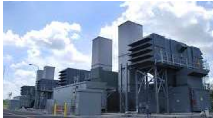
Peaking Gas Turbine
