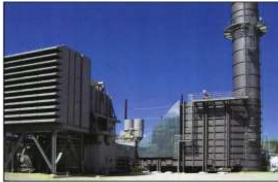
LMS100 Gas Turbine Generator with Encased Clutch at Calpine (formerly Conectiv) Cumberland Energy Center, Millville, NJ.
