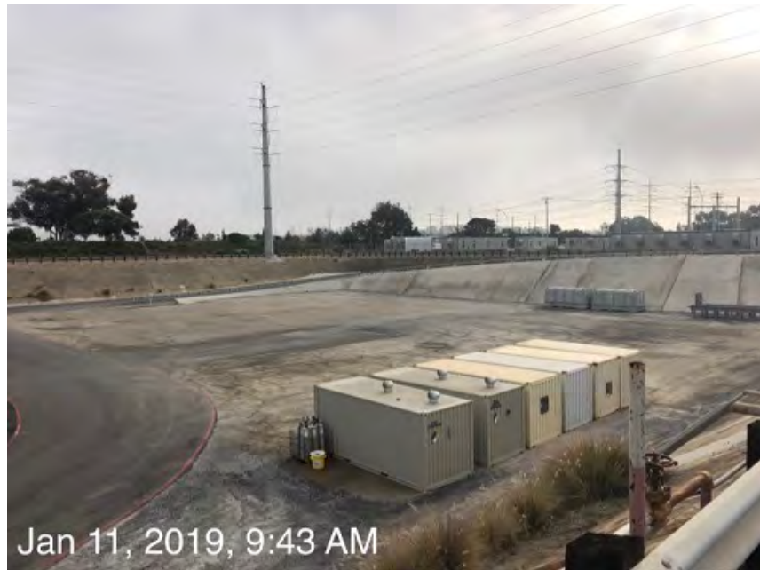
Photo 3. Stored equipment within the Construction Site has been removed as construction is nearing completion. Photo taken 1/11/19, facing southeast.
