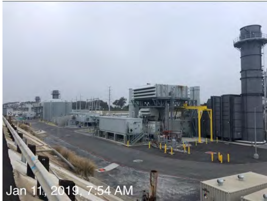
Photo 1: NRG construction is in the final stages of completion. Photo taken 1/11/19, facing northeast.
