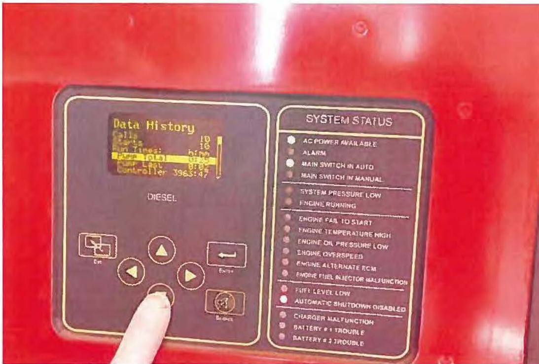
S-6 Controller, Showing Fire Pump Operating Hours
