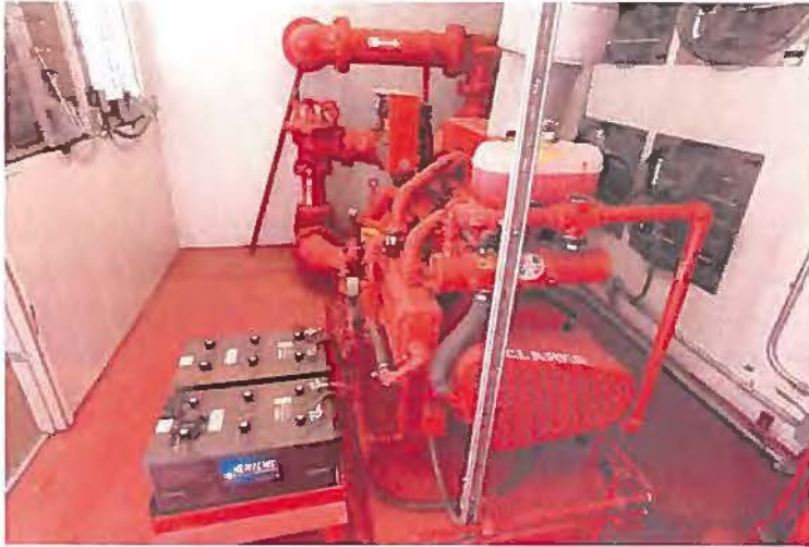
S-6 Emergency Fire Pump
