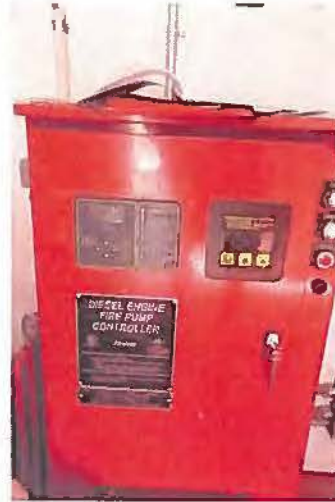
S-6 Control Unit
