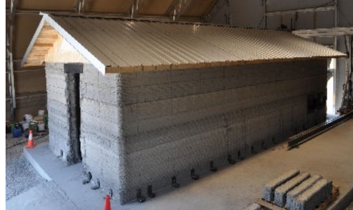
Figure 3. The U.S. Army Corp of Engineers has used 3DCP equipment to print a concrete building in 24 hours.
