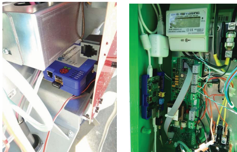
Figure 6- Raspberry Pi Integrated with EVSE (left) and Meter (right- without cover)
