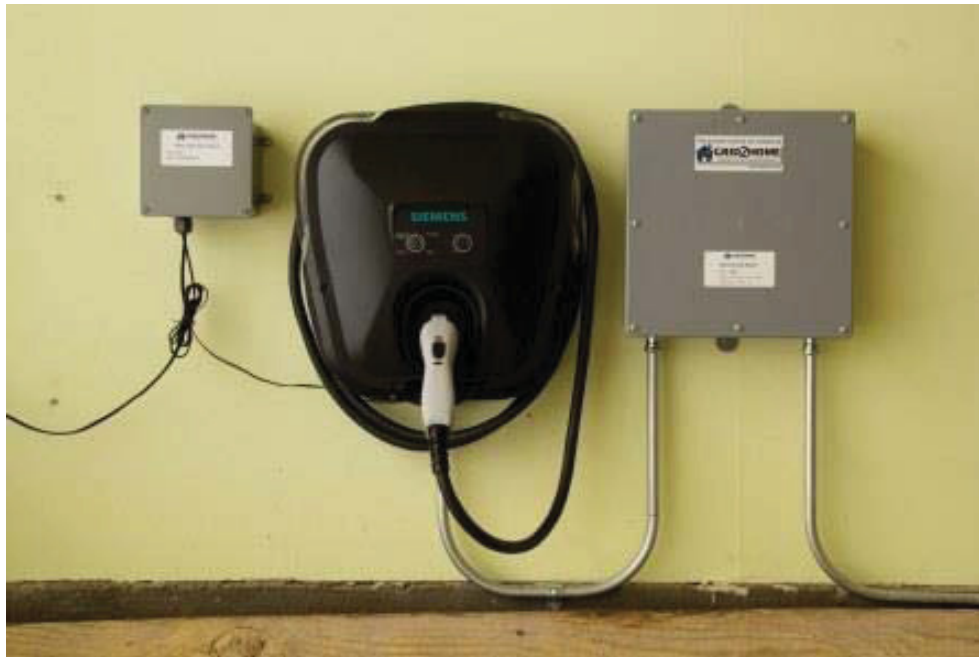
Figure 7- In this customer installation, the EVSE did not have enough space to place the Raspberry Pi (left) inside. The sub-meter on the right could be placed anywhere on the branch circuit, including next to the panel. This unit had a relay allowing only on/off capability (the small wire from the Raspberry Pi to the EVSE).
