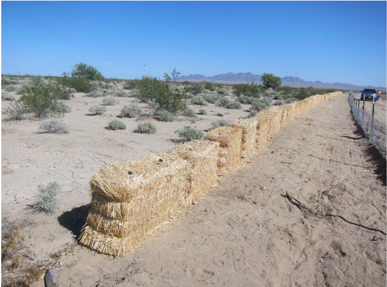
Figure 4 - Stormwater BMPs installed along NE portion of fence
