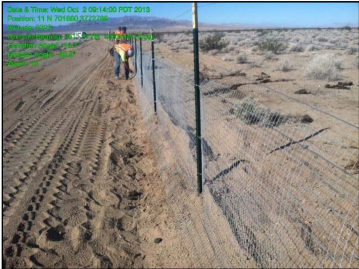
Figure 2 - Desert Tortoise Fence with Backfill
