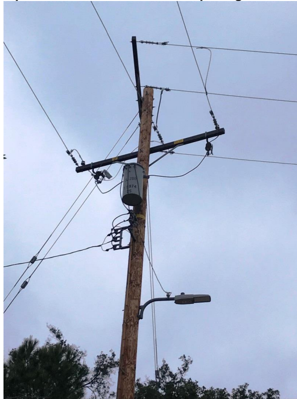
Figure 45: Example of Increased Conductor Spacing in LADWP Territory
