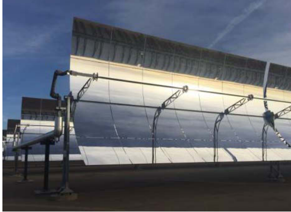
(a) Solar Collector Assemblies (SCAs)
