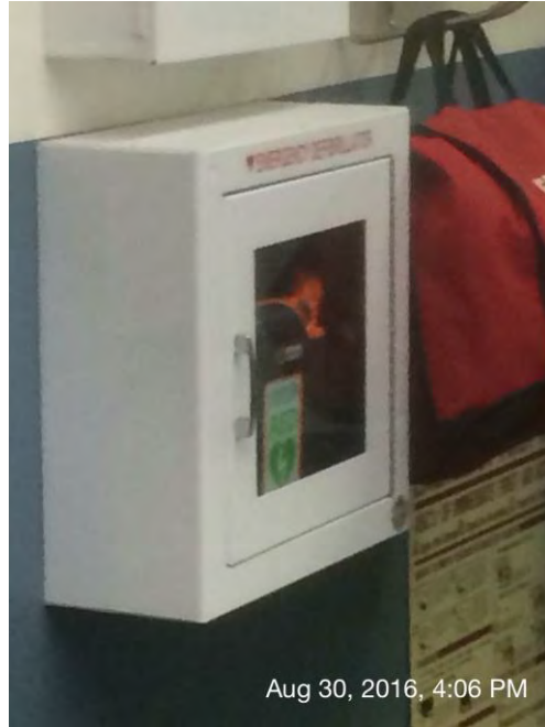
Location: Unit 3 and 4 Control Room
