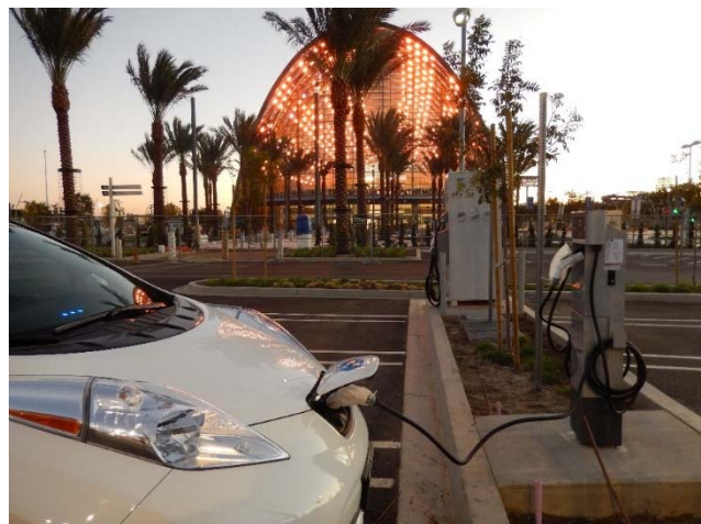
Photo 6: Charging Stations at Anaheim Regional Transportation Intermodal Center
