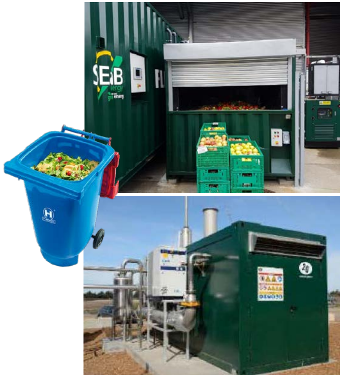
Containerized digester Flexibuster at the Navy Base Ventura County
