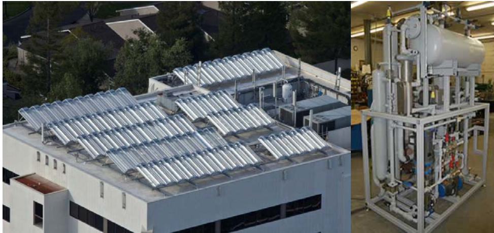
a. Solar thermal and absorption chiller to provide hot water and cooling at a hotel
