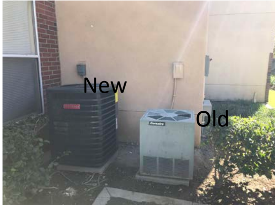
a. High efficiency heat pumps in multifamily retrofits
