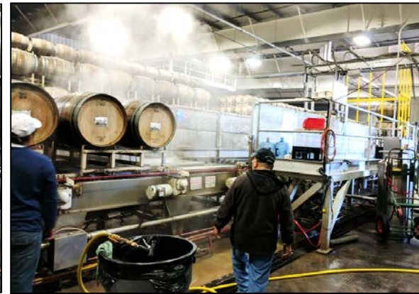
Winery water reuse and energy savings
