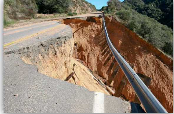
State Route 330, San Bernardino County, Dec. 27, 2010 Photo: California Department of Transportation
