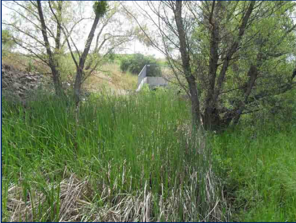
FIGURE 3 Looking south toward culverts at Viera Avenue. Cattail wetland is within the creek channel, and red willow is along the banks.
