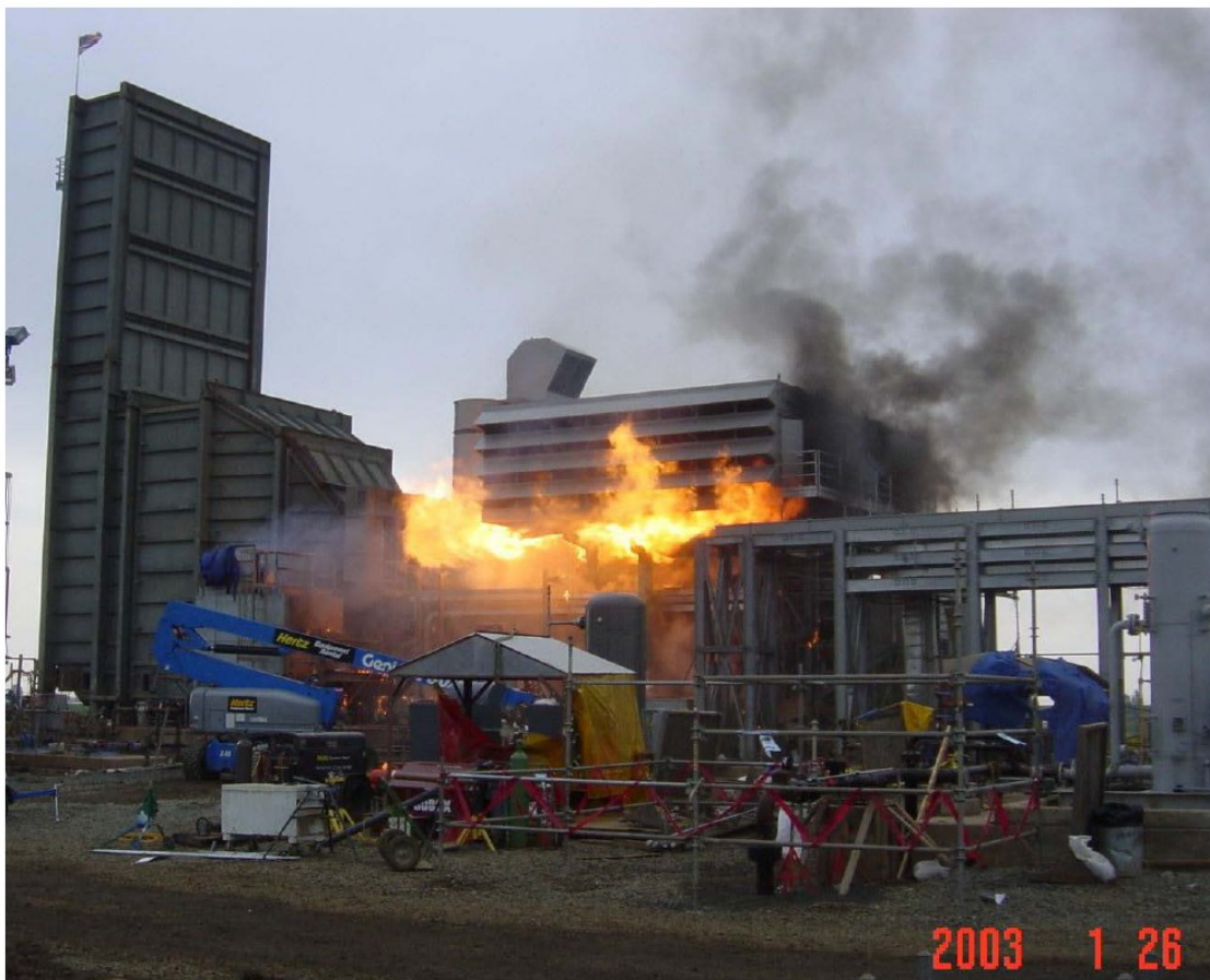
Figure 4. Previous explosion during a natural gas blow on January 26, 2003, at a Calpine natural gas power plant in Fairfield, California. The explosion was heard 10 miles away.
