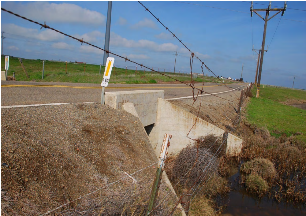
#4. Water line alignment near Drainage 3 (D-3), looking north. The pipeline will be installed under the concrete box culvert by pipe ramming.
