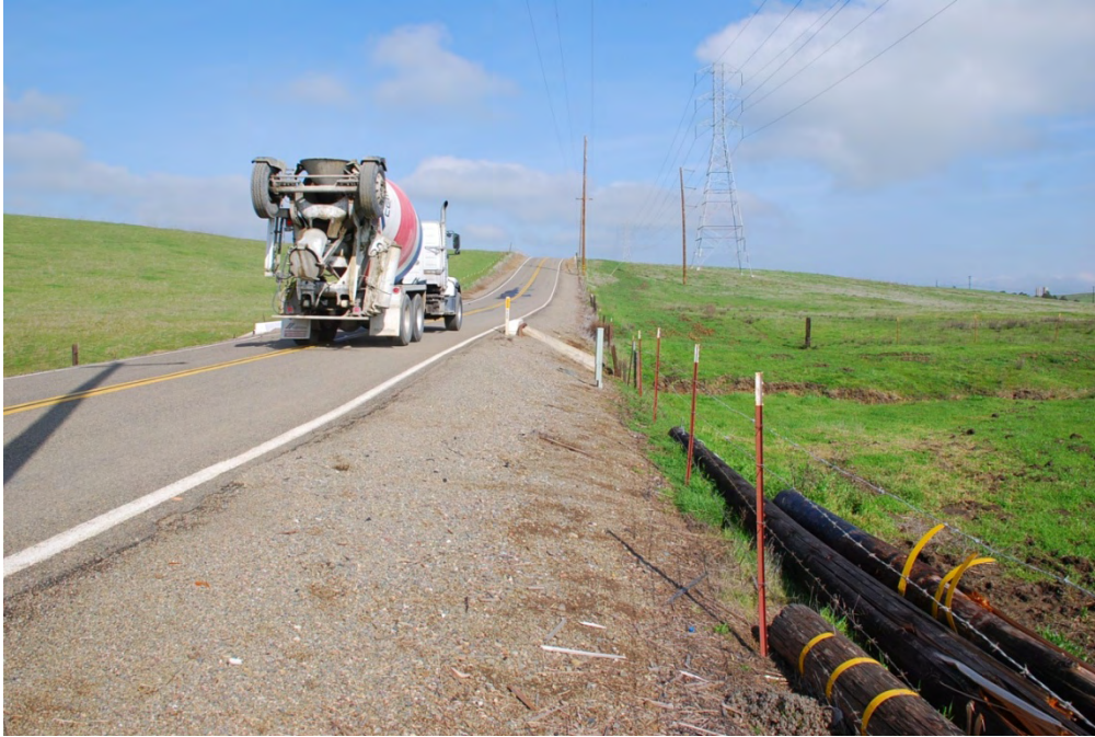
#1. Proposed water line alignment near Drainage 1 (D-1), looking north. The barbed wire fence marks the right-of-way boundary where water line work will be confined to.
