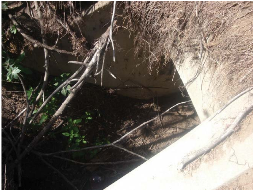
Photograph 2: Looking northeast at culvert that connects drainage ditch to San Jose Creek. Note: this is the only potential federal water that occurs within the survey area.
