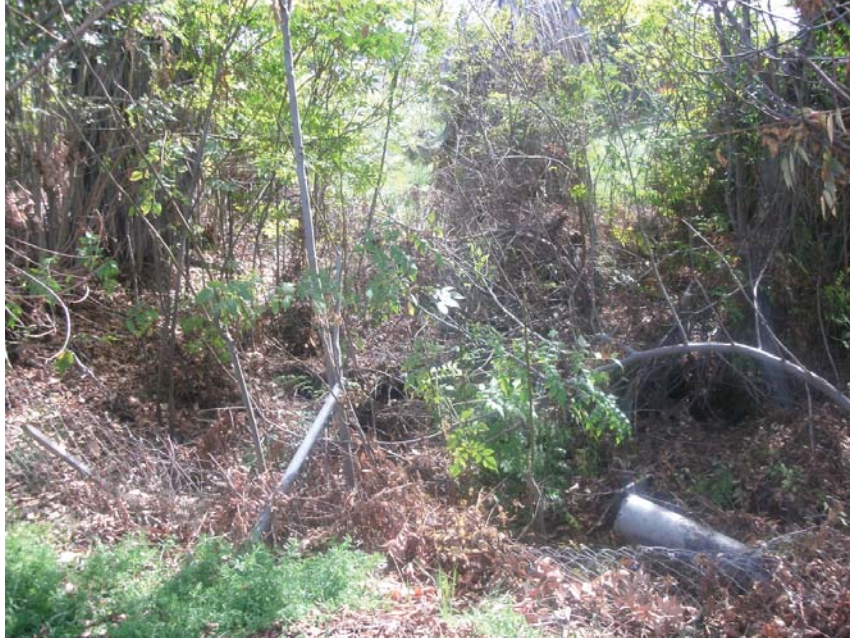
Photograph 3: Looking southwest at constructed swale at compacted dirt service road. There is no culvert connecting this constructed swale to the drainage ditch. Note: area is populated by upland vegetation and debris.
