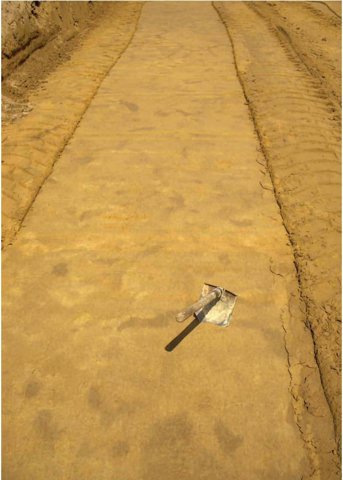
FIGURE DR19-1 MODESTO FORMATION ALMOND 2 POWER PLANT CERES, CALIFORNIA
