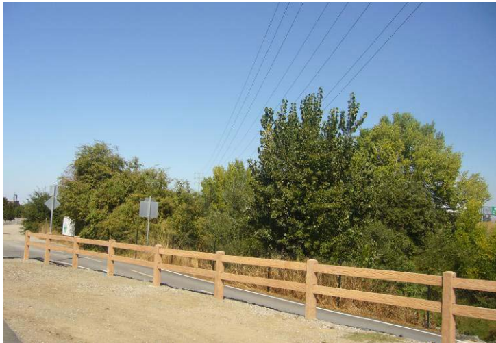
7. Another view of the central portion of the reconductoring project, looking north-northeast along the Guadalupe River. The lines here span across the Guadalupe River riparian
