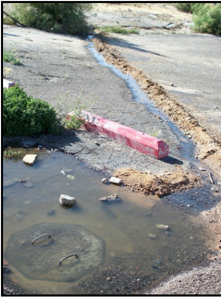
Photo 1: Sewage flow guided by dirt berm, leading to north side of parking pavement.
