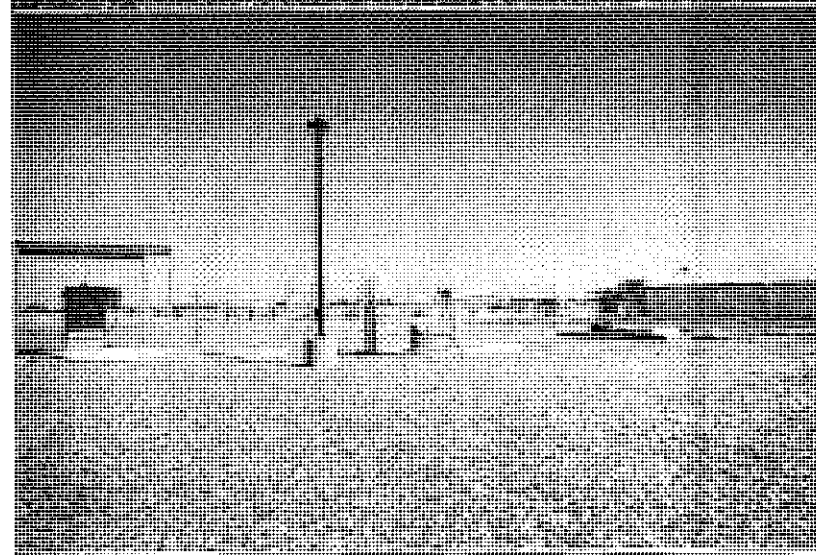
Photograph 6 - Mudline Monitor, influent pump station, septic tank drop cell, and flow meters located north of aeration ponds.
