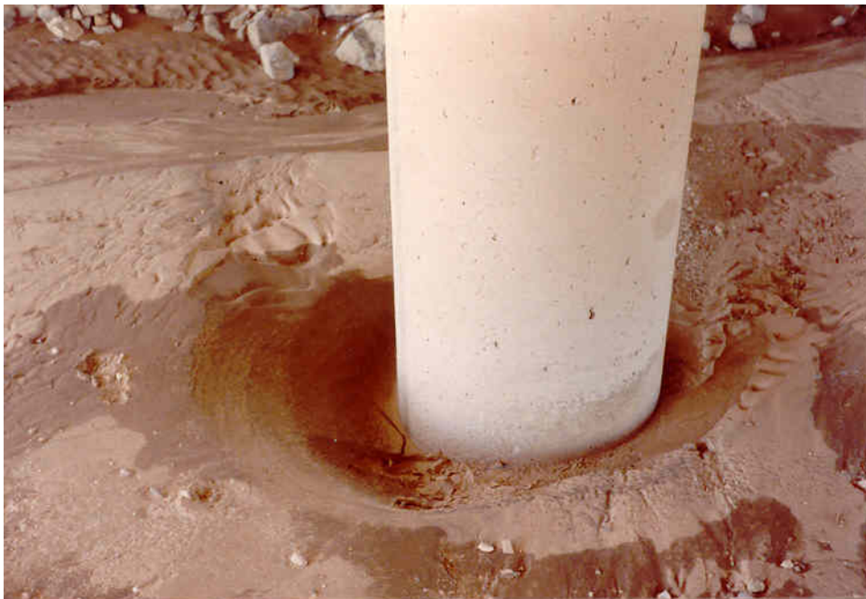
Figure 1. Local scour around bridge pier
