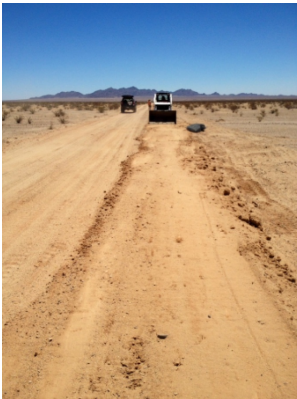
Photograph 2 - Final grading of the tortoise fence area along the south perimeter using the bobcat, facing east
