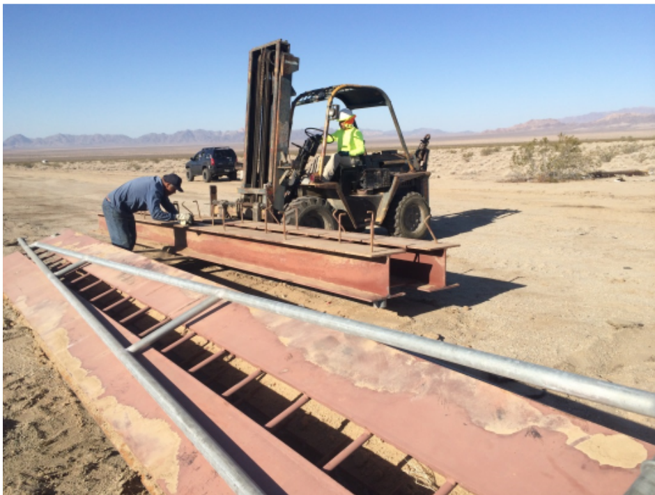
Photograph 4 - Tortoise exclusion guards being removed and staged prior to being hauled offsite.
