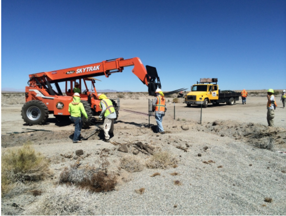
Photograph 5 - Last section of tortoise fence removed at the entrance to the site.
