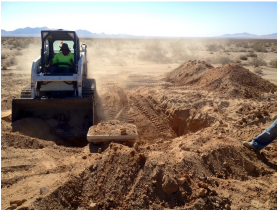
Photograph 6 - Excavations around the large footing that held the meteorological tower (depth of approximately 5 feet) before dislodging it and dragging it out, facing southeast.
