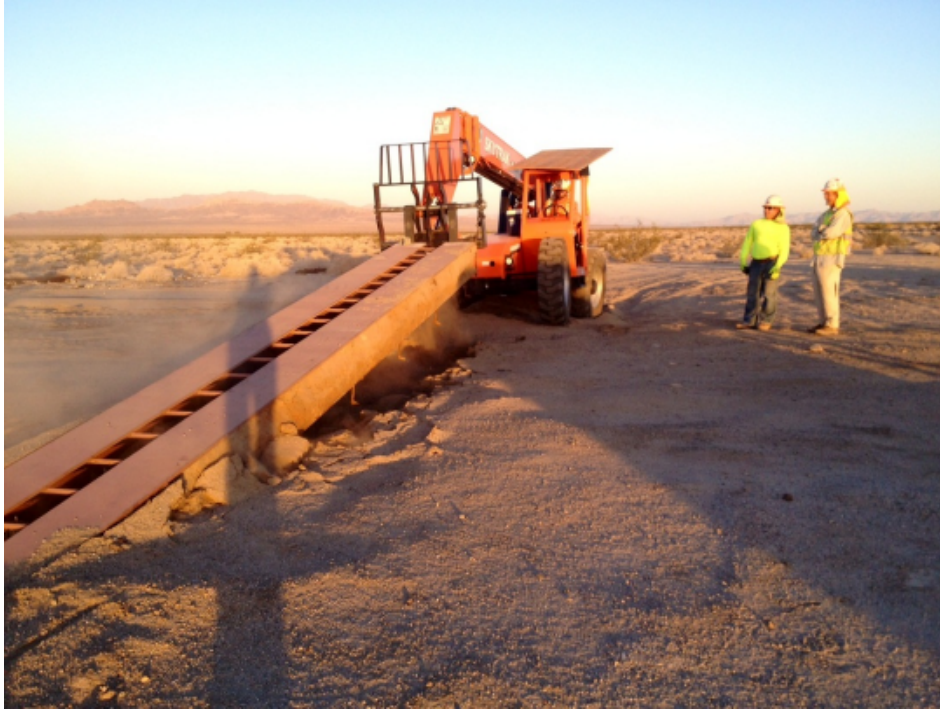
Photograph 3 - Tortoise crossing guards were removed and trenches were backfilled along the northern perimeter where entry gates had been located, facing east-northeast.
