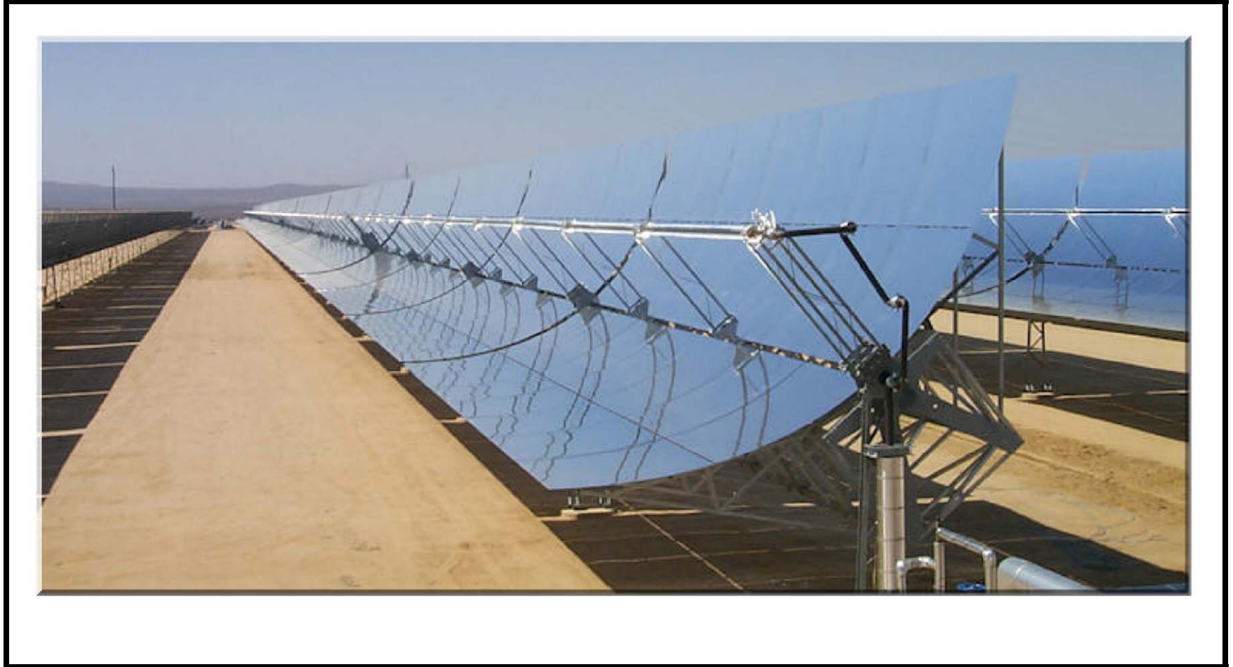
Figure 6: Picture of Trough Solar Collector
