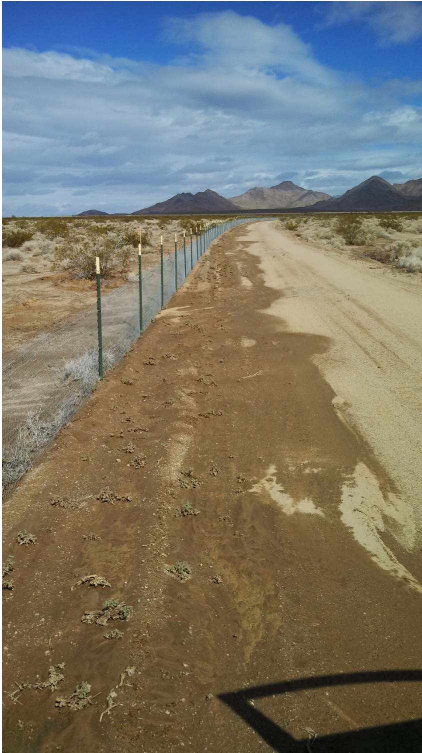
TYPICAL RUNOFF PATTERN ALONG THE MAJORITY OF THE WESTERN FENCELINE (BETWEEN LOCATIONS 2 AND 6). VIEW NORTH
