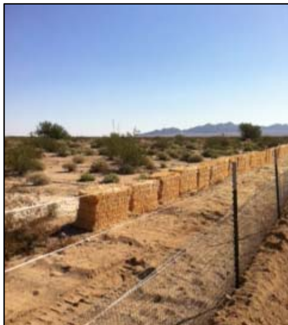
Figure 8 - RSEP Site Erosion Control BMPs
