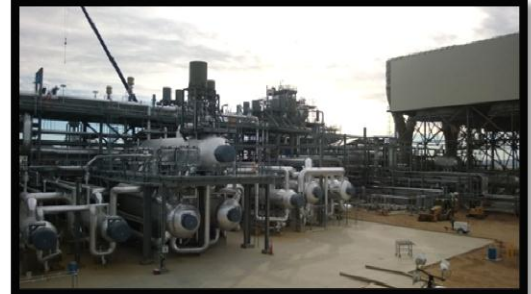
Power Block 1 – Train 1
