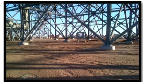
Power Block 1 – ACC
