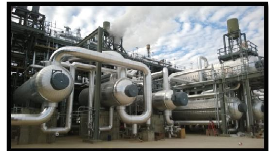
Power Block 1 – Train 2
