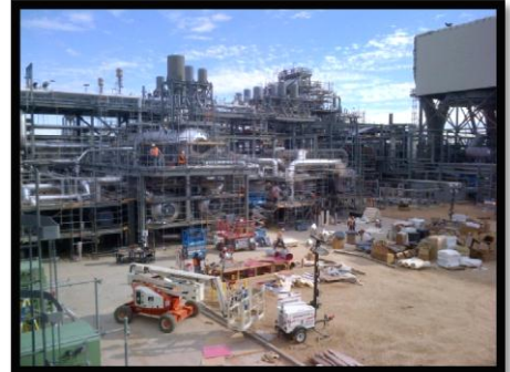
Power Block 1 – Train 1
