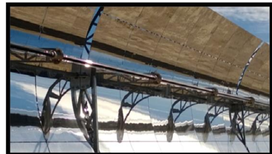
Solar Field 1 – Block 1
