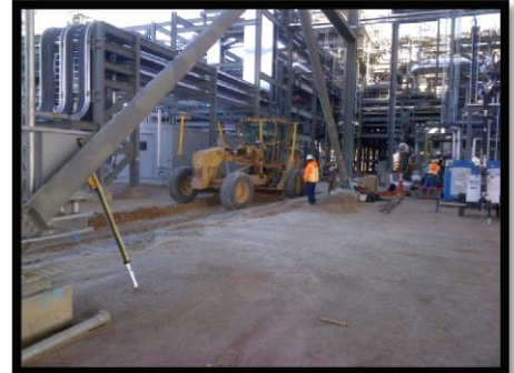
Power Block 1 – ACC
