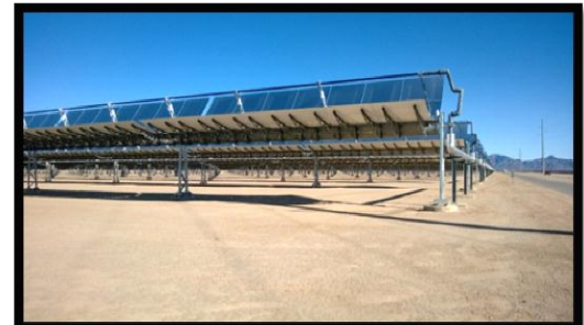
Solar Field 1 – Block 8
