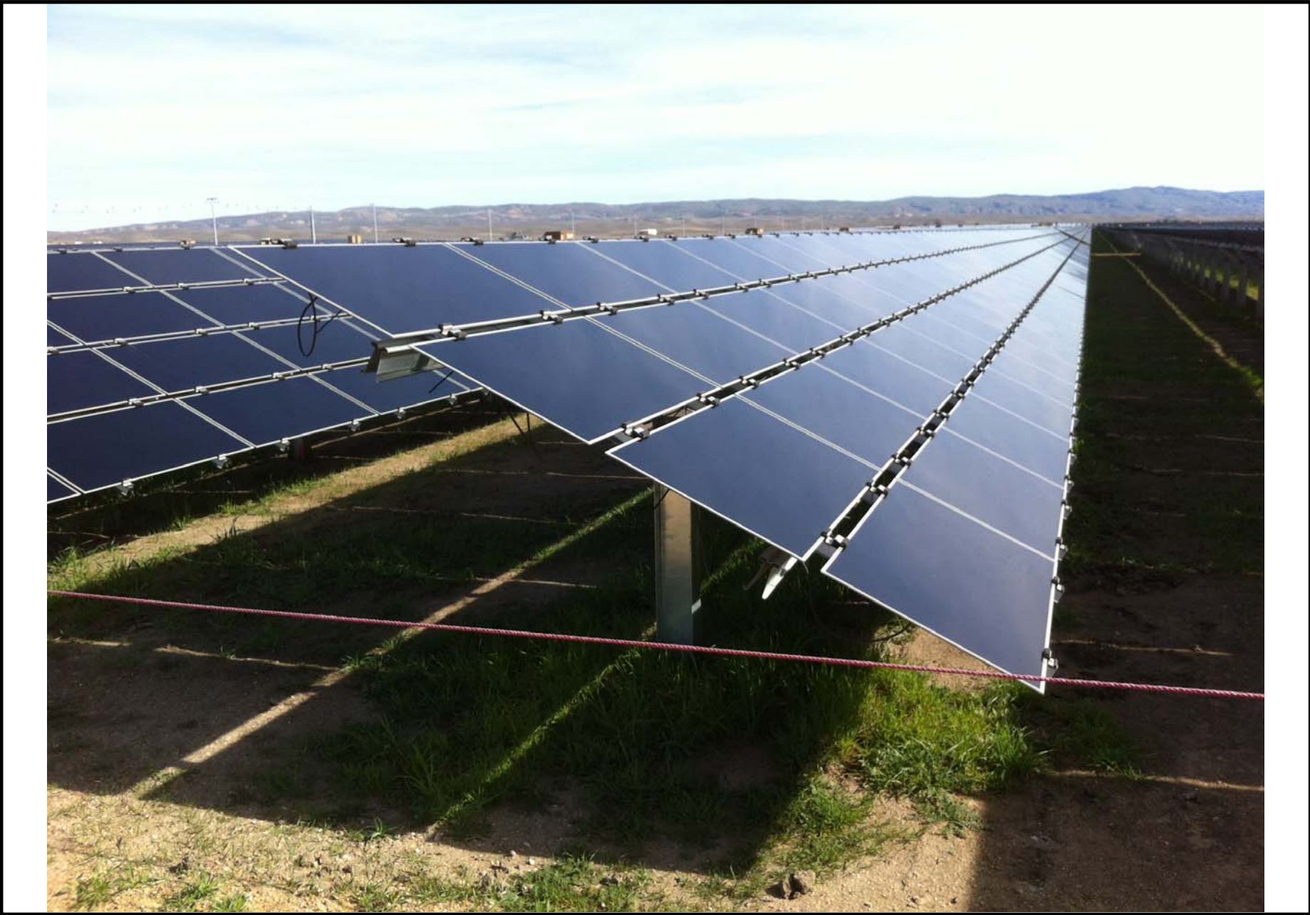
Hidden Hills Solar Electric Generating System (HHSEGS) - Site Preparation and Revegetation at the Topaz Solar Farm Project Site - PV Array Block 6 after Construction
