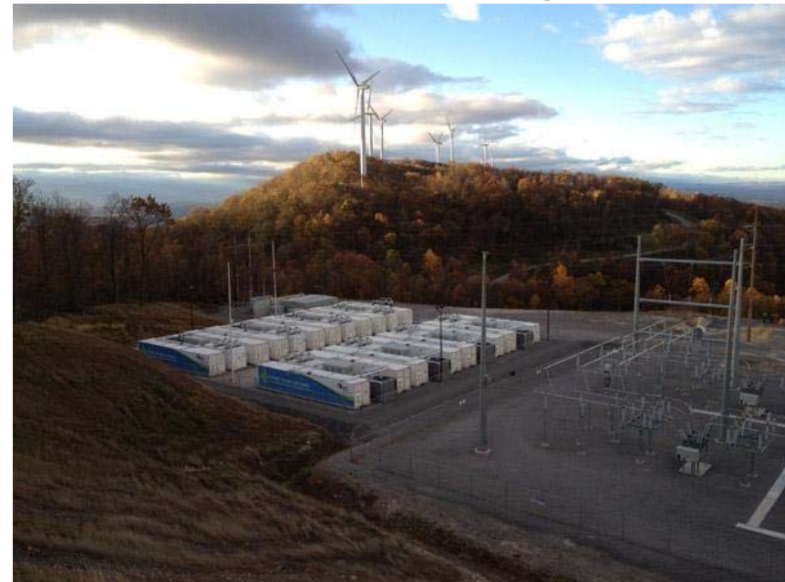
32 MW lithium battery array, 98 MW wind farm, West Virginia
