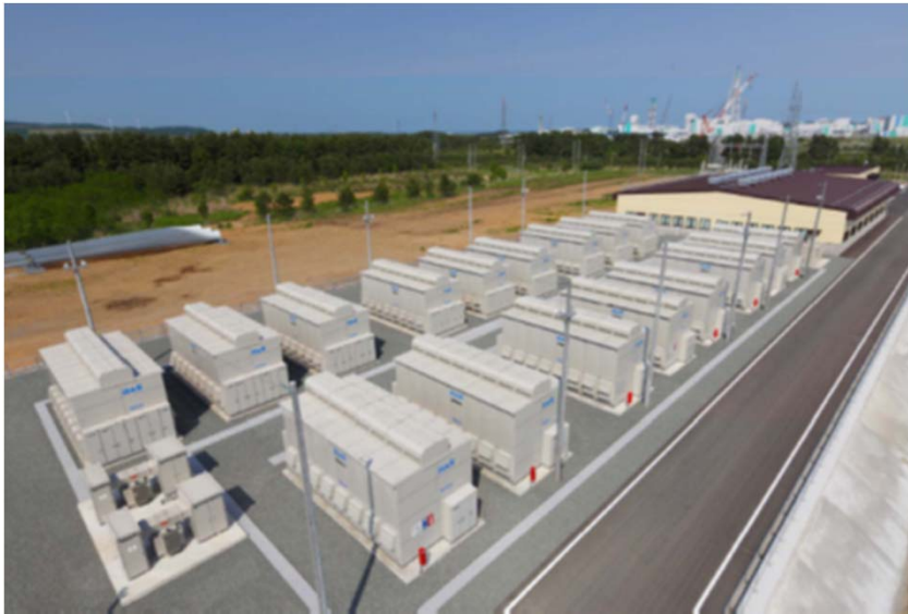
34 MW NaS battery array, 51 MW wind farm, Japan
