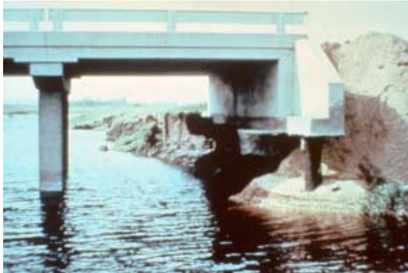
Figure 7.2. Scour of bridge abutment and approach embankment.
