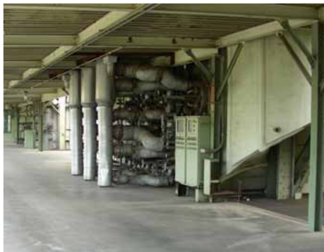
Photograph 6. Unit 3 boiler feeder, camera facing northeast
