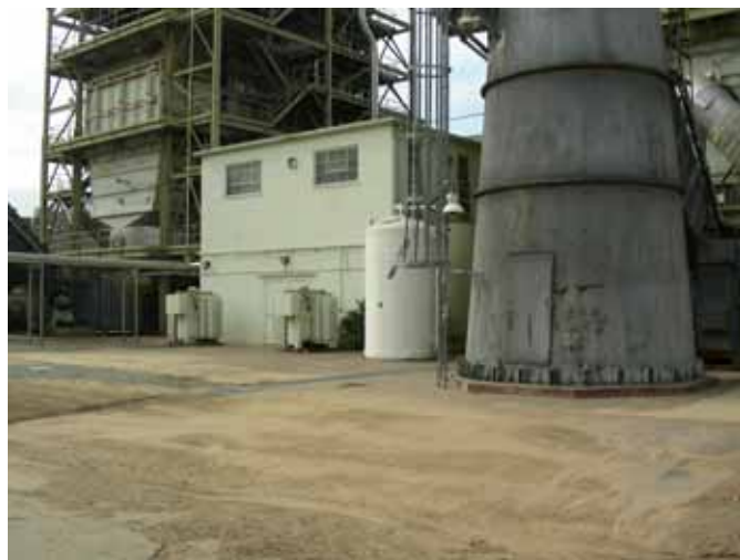
Photograph 8. Unit 3 & 4 Control room, camera facing west
