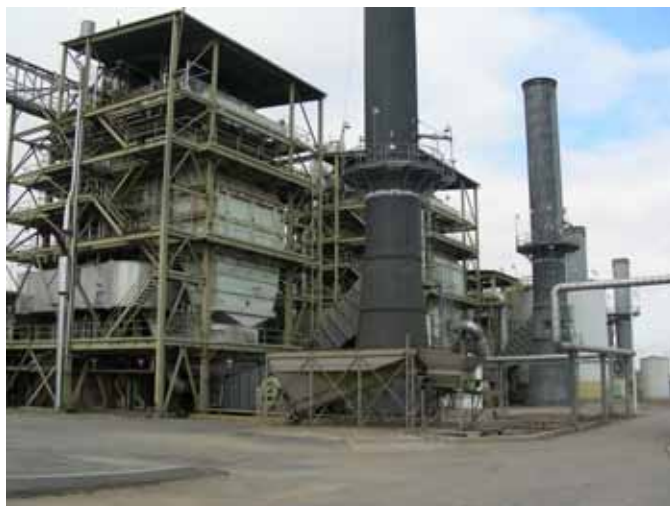
Photograph 4. Boilers, flues and stacks, camera facing northwest
