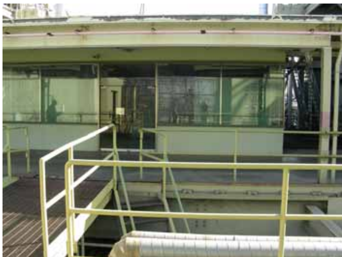
Photograph 7. Unit 1 & 2 Control room, camera facing east
