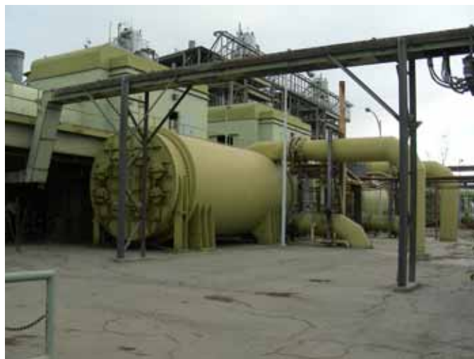
Photograph 12. Hydrogen cooling tank, camera facing southeast
