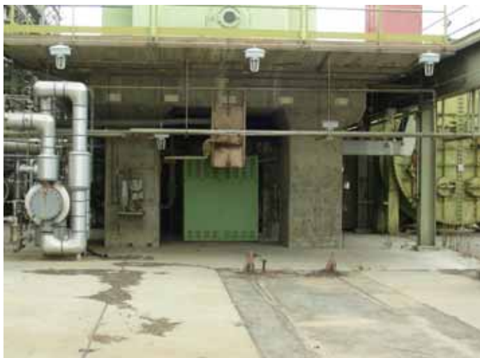
Photograph 11. Unit 1 turbine, camera facing north.
