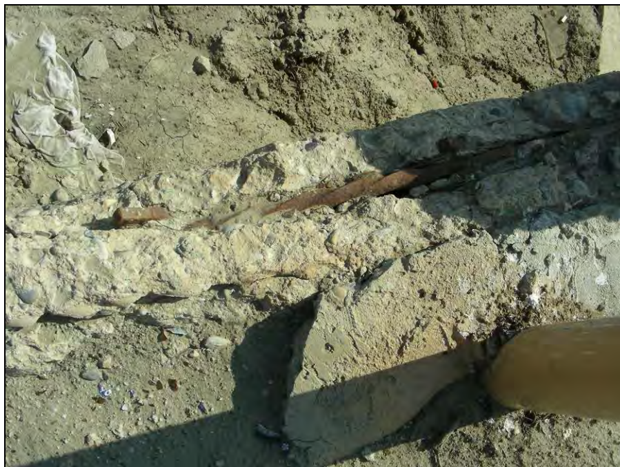
Photograph 11: 2009 view of exposed twisted rebar.
