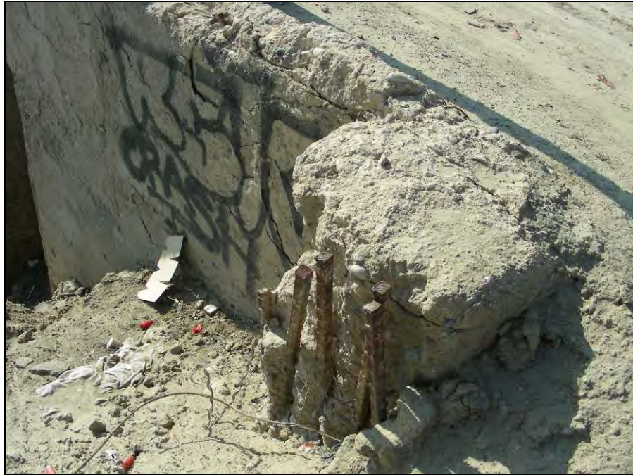
Photograph 10: 2009 view of exposed notched rebar.
