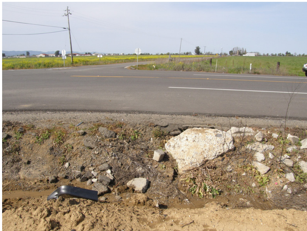
PHOTO 16 AD-07, Possible Obscured Outfall to the Eastern Primary Drainage, to the North. (March 17, 2009)
