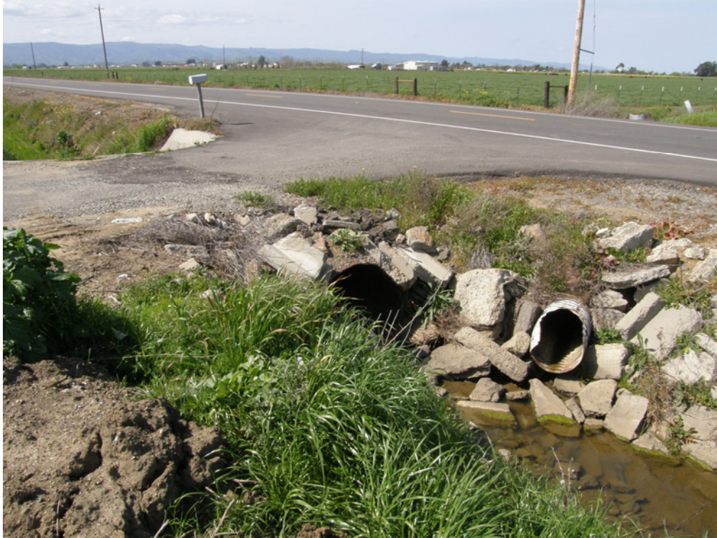
PHOTO 25 AD-14, Showing Outfall to the Eastern Primary Drainage, to the Northwest. (March 17, 2009)
