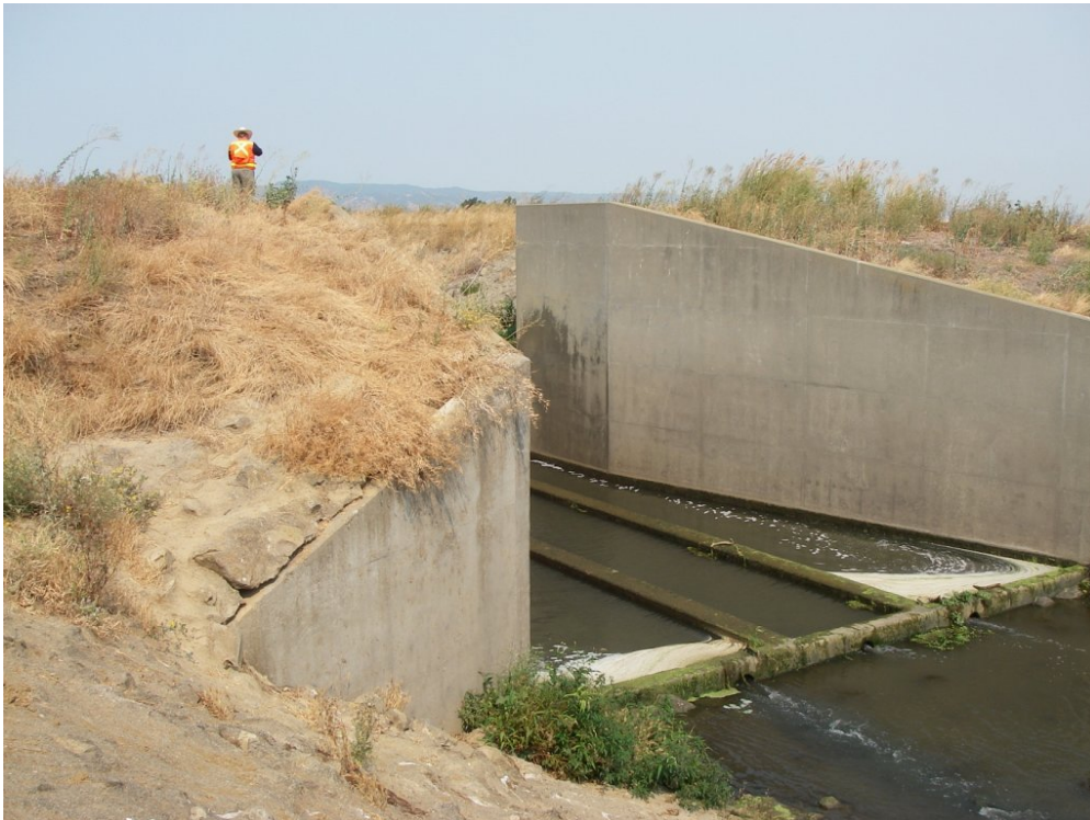
FIGURE 4-4 Grade Control Structure at New Alamo Creek Looking at the Downstream End of the Structure (semi-submerged concrete walls shown in bottom right)
