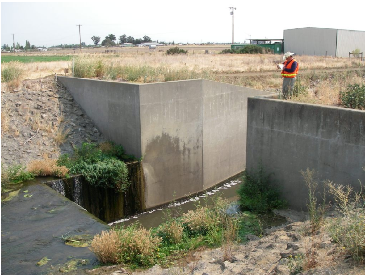
FIGURE 4-2 Grade Control Structure at New Alamo Creek at RM 4.2 (vertical drop in foreground on far left)
