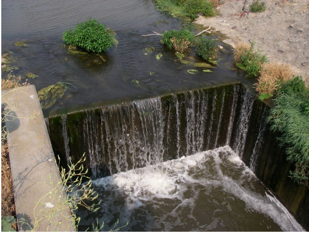
FIGURE 4-3 Grade Control Structure at New Alamo Creek Looking Upstream (at vertical drop in middle of photograph)
