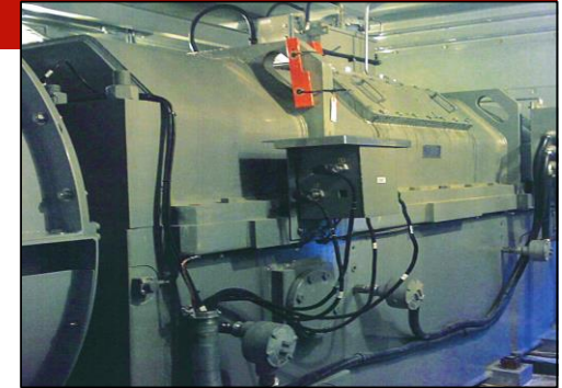
130 MW rated Size 272T SSS® Encased Clutch installed in LMS100.
