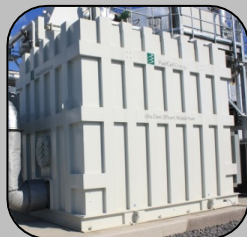
Completed Module 1.4 megawatts
