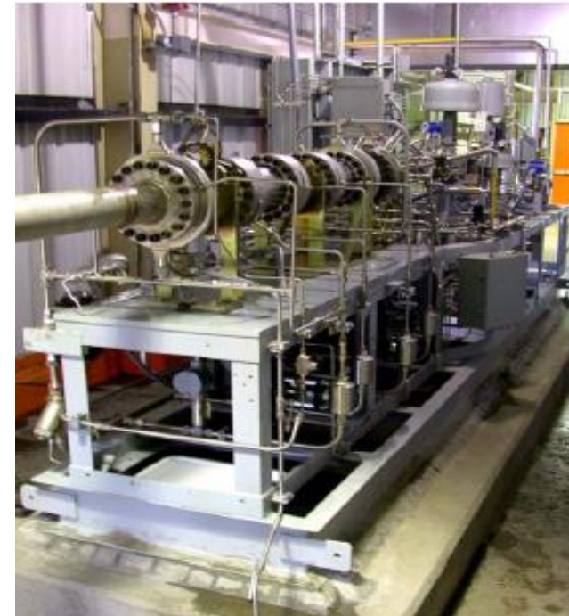
20MW t Gas Generator
