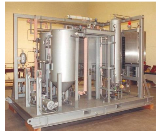
Skid-mounted HTP system
