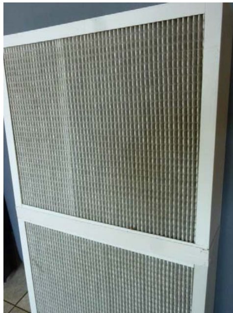
Figure 88: MERV 16 Filter Installed at House 10
