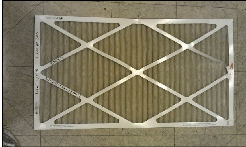
Figure 21: Original Filter Found in Furnace at House 3
