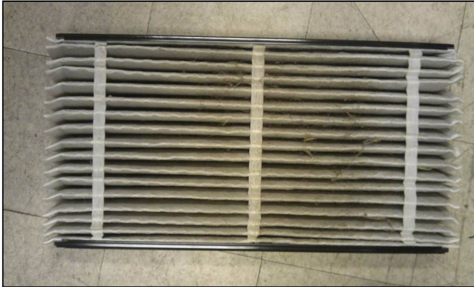
Figure 69: Dirt Accumulation on Flexible Pleated Filter in House 8
