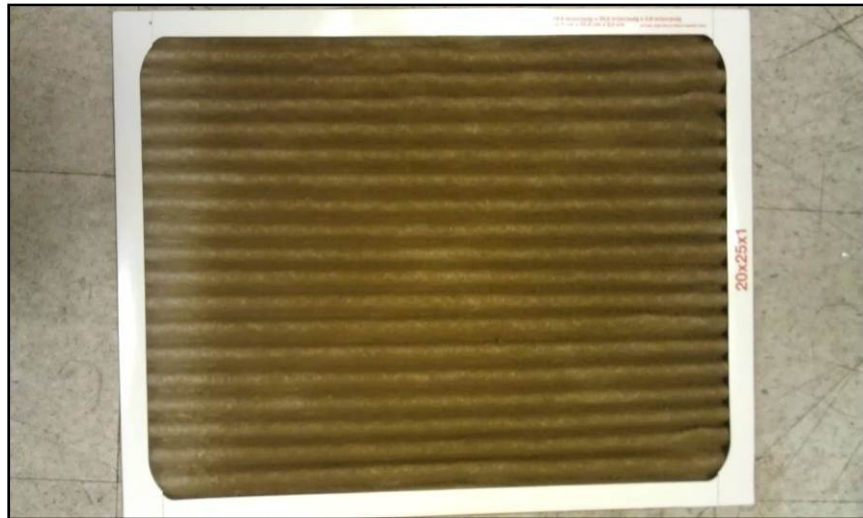
Figure 58: Original Furnace Filter Installed in House 7
