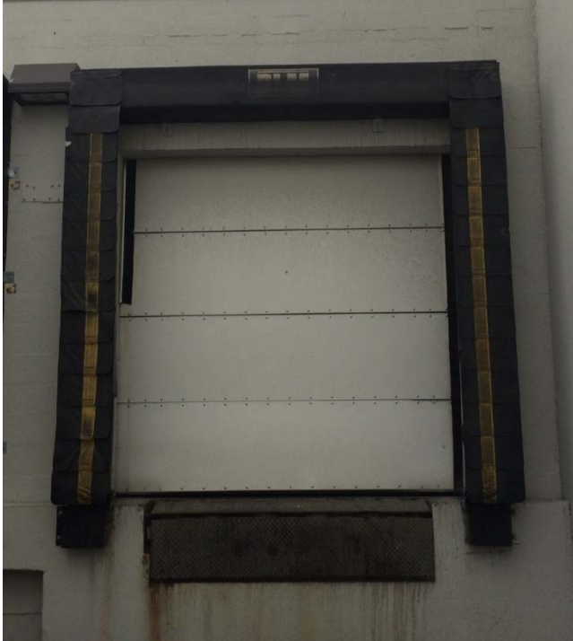
Figure 1: Loading dock with seal
