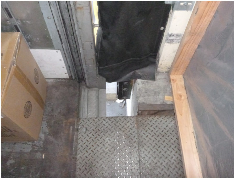
Figure 3: Gap between dock leveler and dock seal
