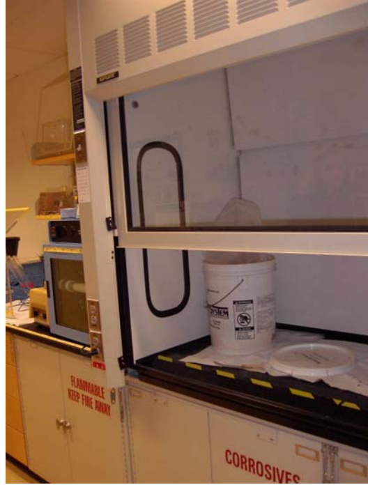
PES Demo hood prior to retrofit (Note sash stop restricts sash opening more than 50%)
