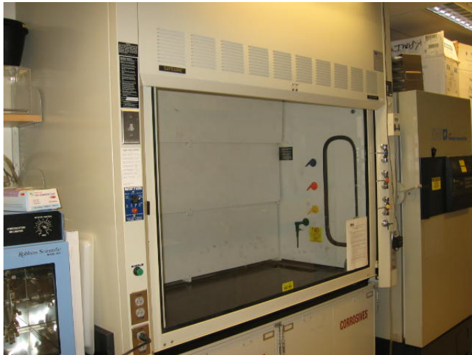
Demonstration Fume Hood in PES 1247 (after installation)
