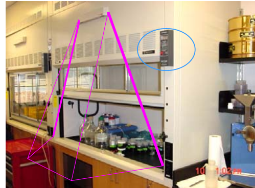
Auto-closure fume hoods with occupancy detection
