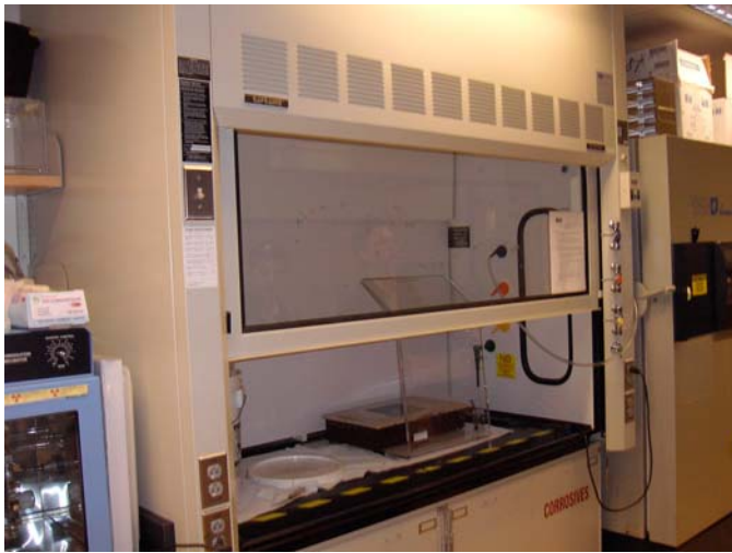
PES hood prior to retrofit with hose that would not allow sash to close
