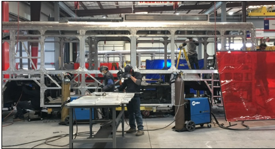
BYD Motors Inc. employees fabricating an all-electric transit bus shell in Lancaster.
