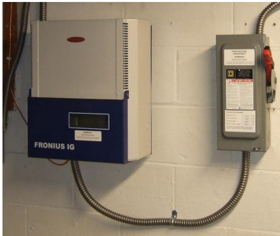
Figure 1: Residential string inverter and manual disconnect.
