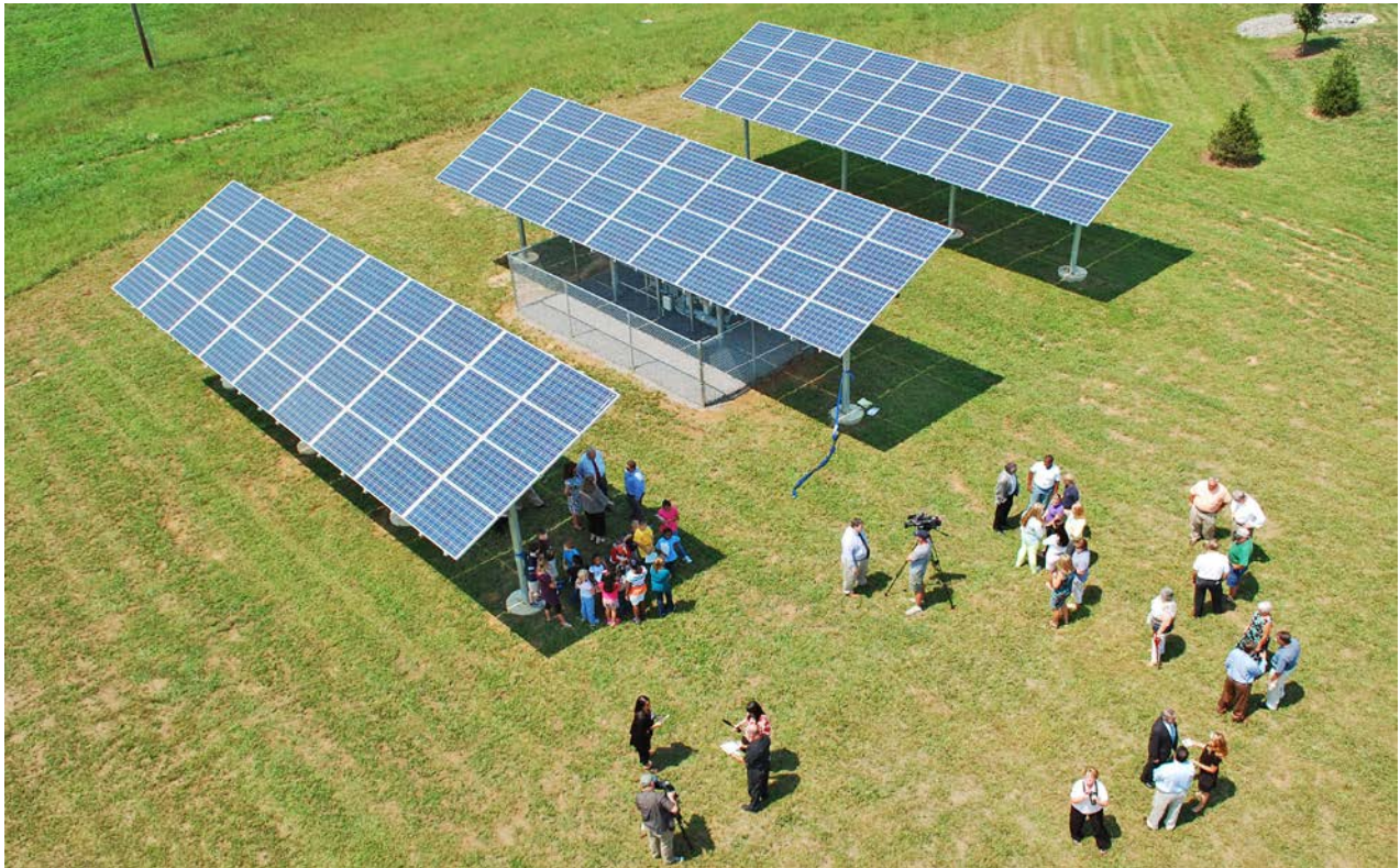
The 2012 ribbon-cutting event for a community solar project at the Duck River Electric Membership Cooperative in Shelbyville, Tenn. (Photo courtesy of Duck River EMC.)
